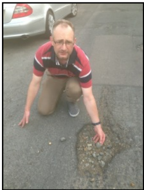
Sean Meiszner checks a pothole in Marten Road
